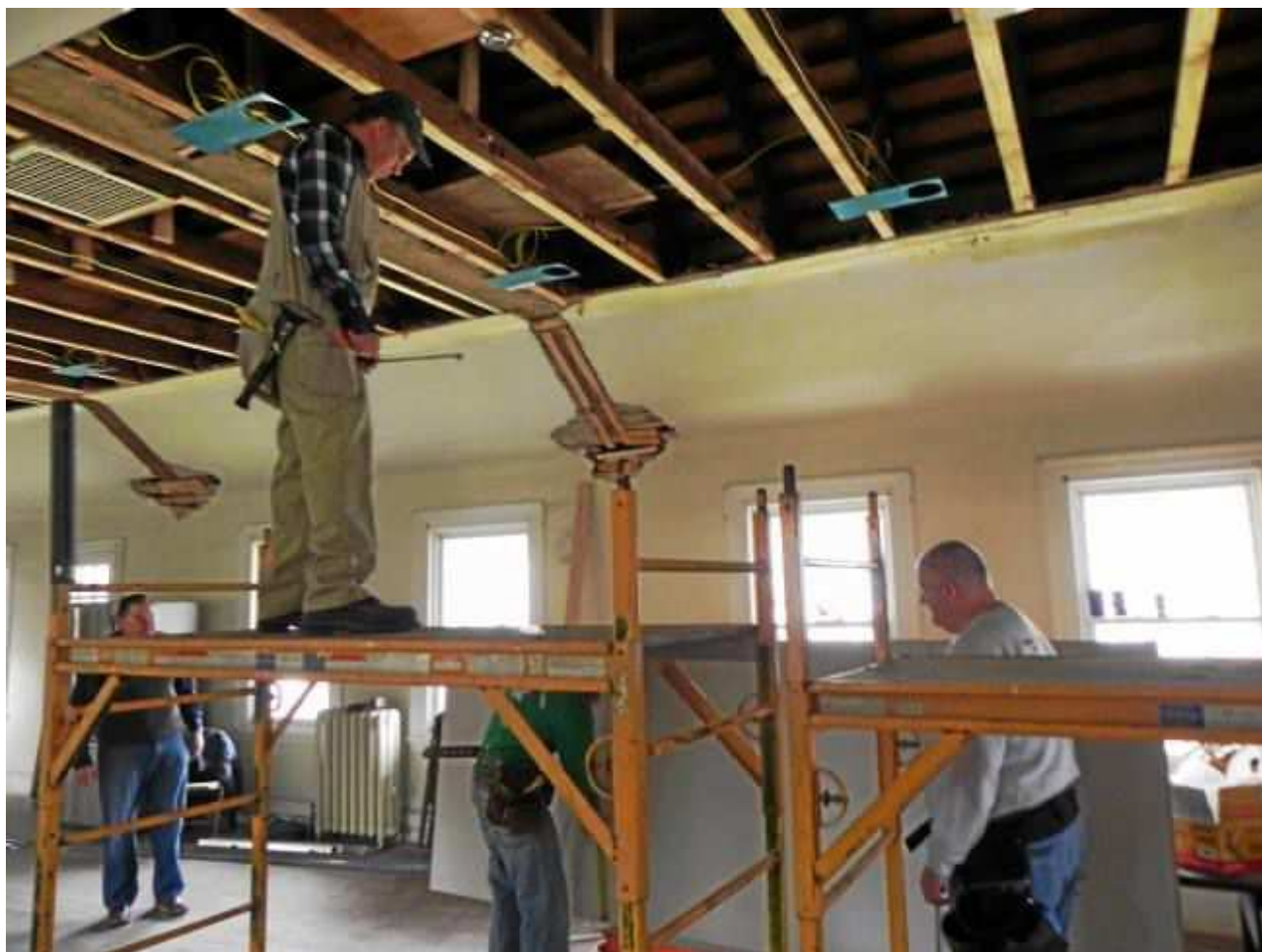
Volunteers working on the Radnor Township Civic Association building. Volunteers work on the Radnor Township Civic Association building.
